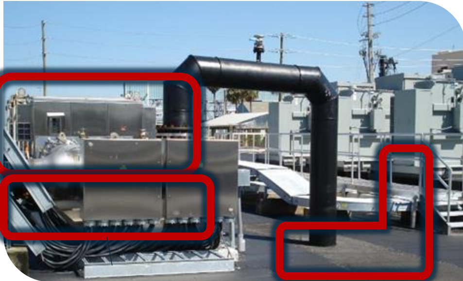
Traditional Low Voltage installation
